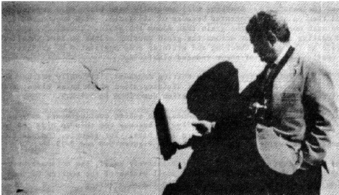
FIGURE 5-2b A Chalky-Masonry Surface
