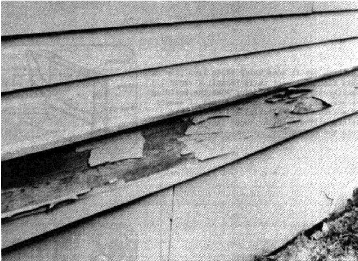
FIGURE 5-33 Moisture Peeling Caused by Contact with Ground
