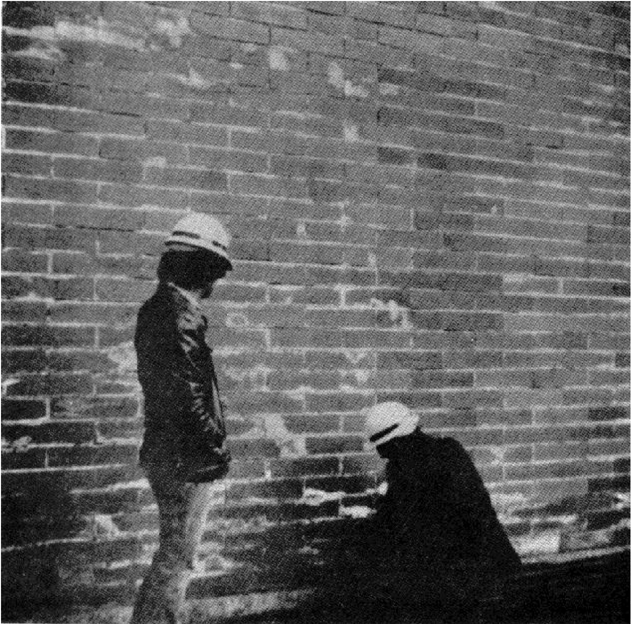
FIGURE 5-19 Severe Efflorescence on Brick Wall
