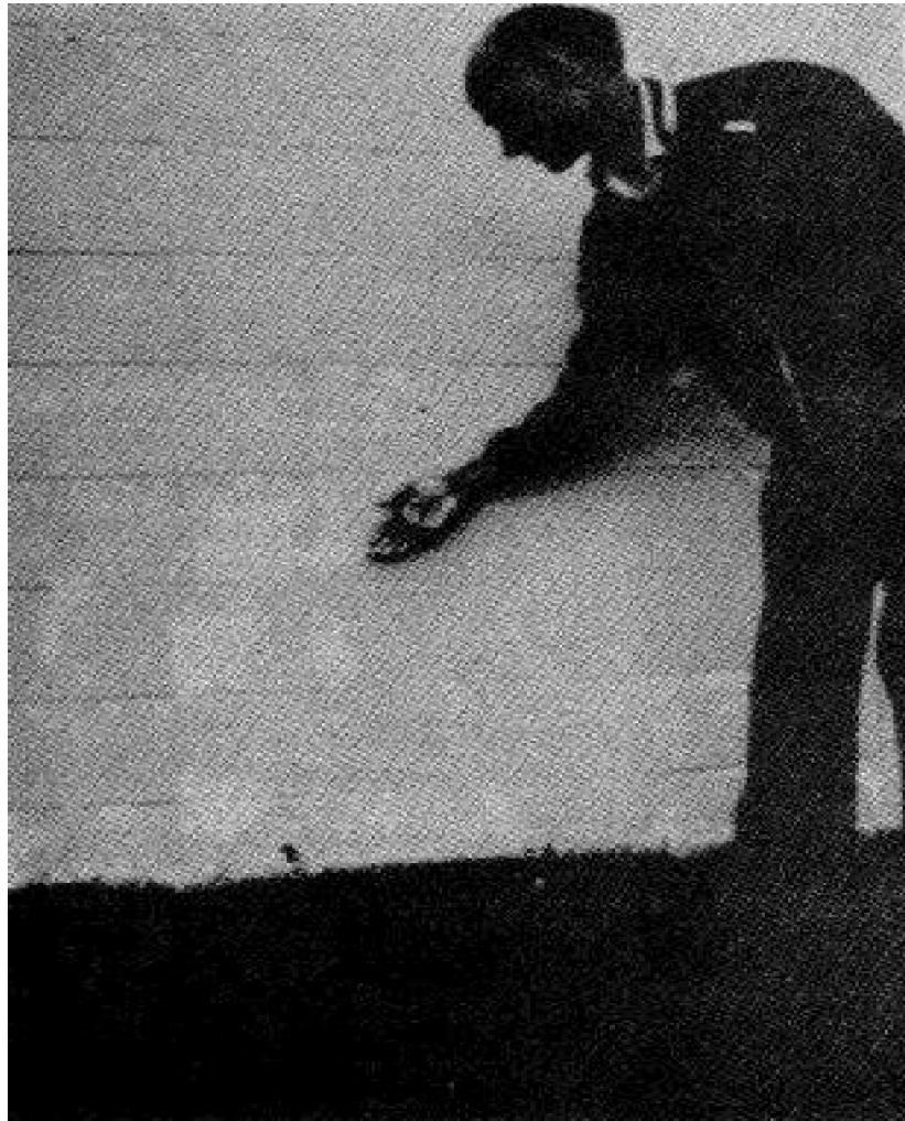
FIGURE 5-3 Failure of Water-Thinned Paint to Adhere to Chalky Surface
